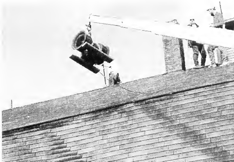
Preston Starr, Steve Obermiller and Steve Hansen save the fire siren from the old IGA during demolition
